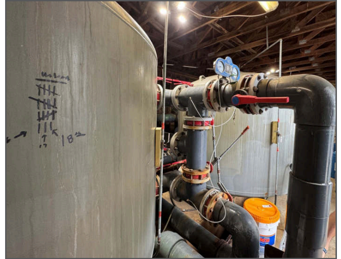
Existing Sand Filters
