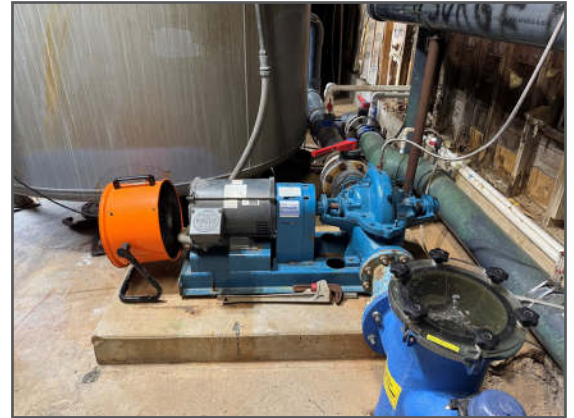
Existing Pool Circulation Pump and Cooling Fan
