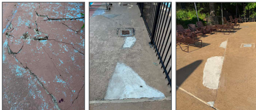
Deck Damage + Repair Efforts
